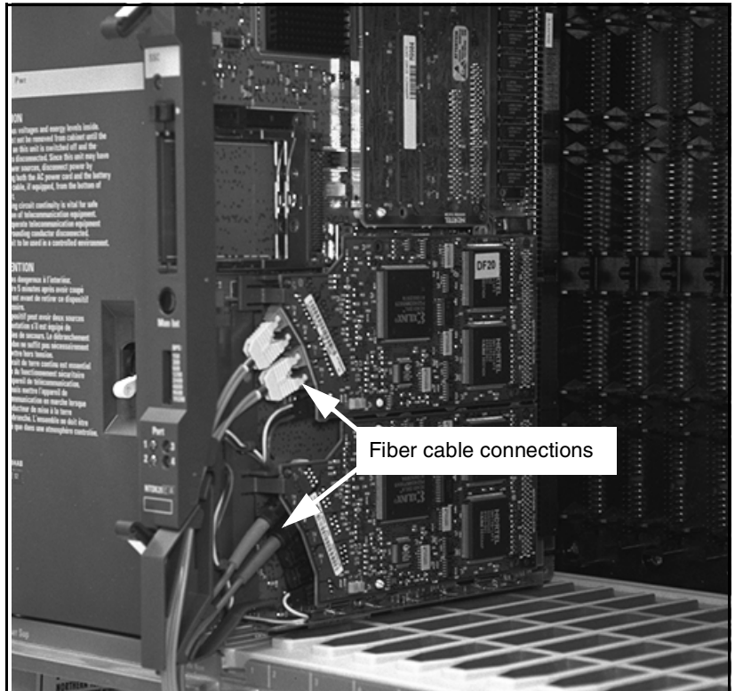
Figure 14 Fiber-optic cable connections
